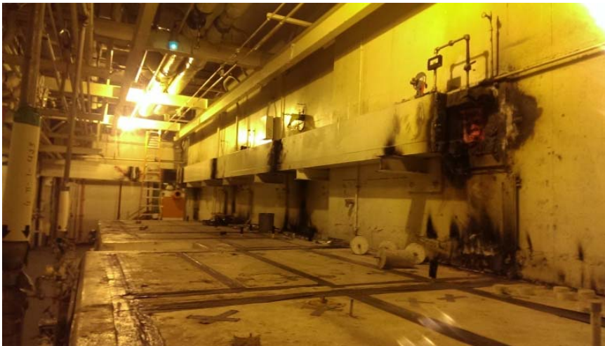
Upper Warm Aisle after Deactivation
